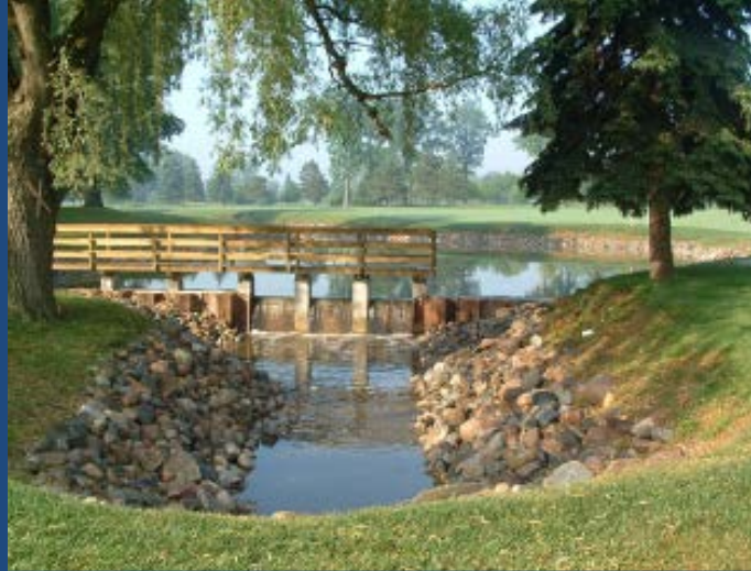
Example- Steel Sheet Pile Structure at Great Oaks Country Club in Rochester, MI.
